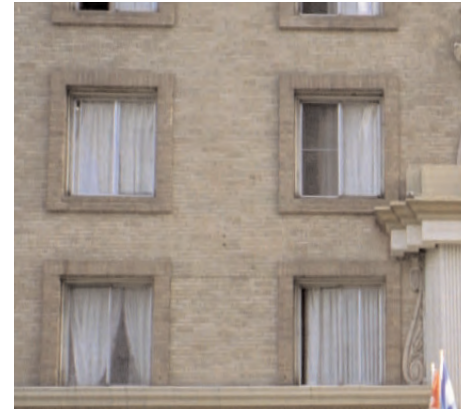
These replacement aluminum windows do not provide the same sense of detail or scale to the building facade as the originals. The lack of window mullions disturbs the facade proportions.
