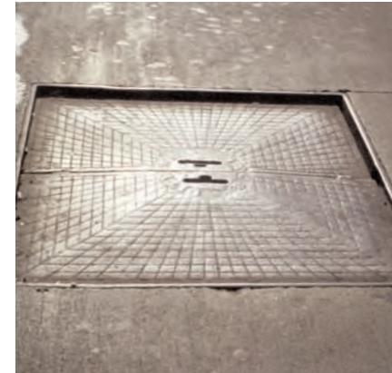
One of the basement hatches on Broadway decorated with a sunburst pattern.
