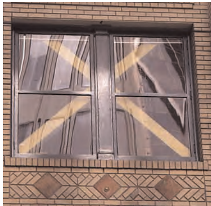
This unreinforced masonry building was structurally upgraded using steel X-bracing. This type of system is often visible from the exterior through windows; care should be taken to design these systems with the least visual impact.
