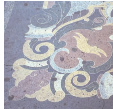
A detail of the terrazzo outside the Los Angeles Theater. The accumulation of gum is evident on the surface.
