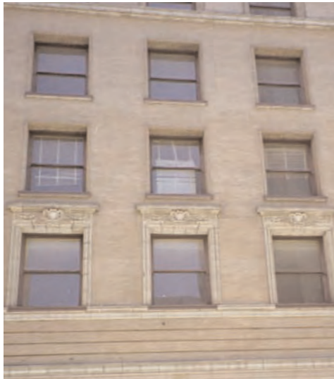
A detail of the Third Street elevation of the Douglas Building showing the terra cotta caps above the windows, the window condition, and the storefront cornice.
