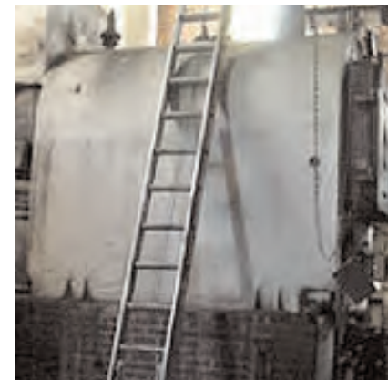
Historic buildings commonly were heated with a boiler and steam heat. These types of systems often must be upgraded during rehabilitation.
