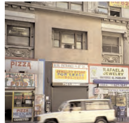
This facade addition to the second story has changed the emphasis of the building's proportions from horizontal to vertical.
