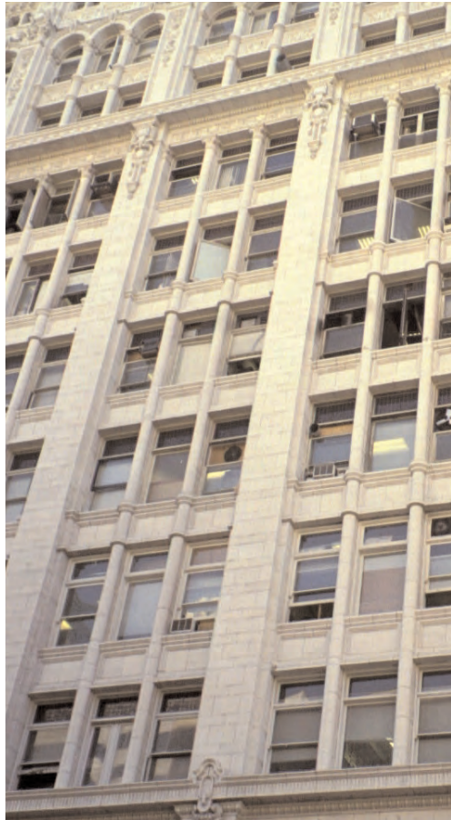
The upper story windows on this building have a number of problems that are common throughout the study area, including sporadically placed air conditioning units, items stored in front of windows at interior spaces, and broken or non-operational windows.
