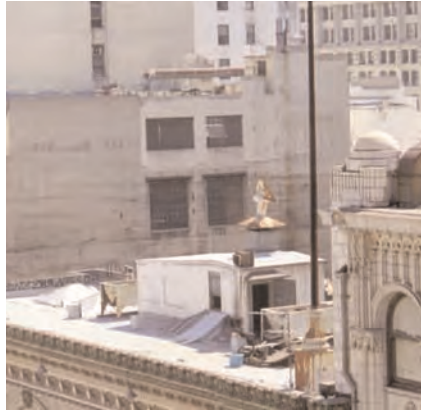
Many rooftops have small penthouses for mechanical equipment or roof stair exits. These features should be retained and reused for roof access and equipment storage; however, roofs should be kept free of excess debris and equipment.
