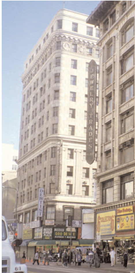
This corner building is a classic three-part commercial building consisting of the base, middle, and top. A phased approach to rehabilitation of this structure could start with the storefronts, then move to the upper stories, including terra cotta and window survey and then repair, if necessary.
