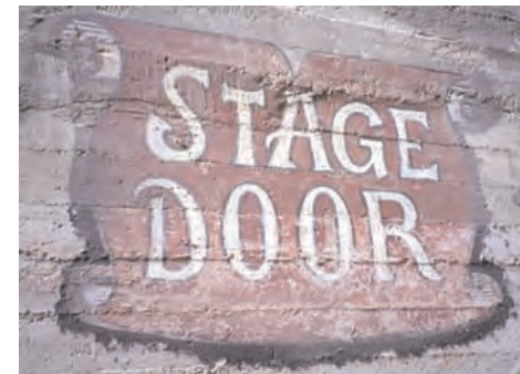
The faded painted stage door sign at the Palace. This type of historic signage is considered a character-defining feature of the building and should be preserved.
