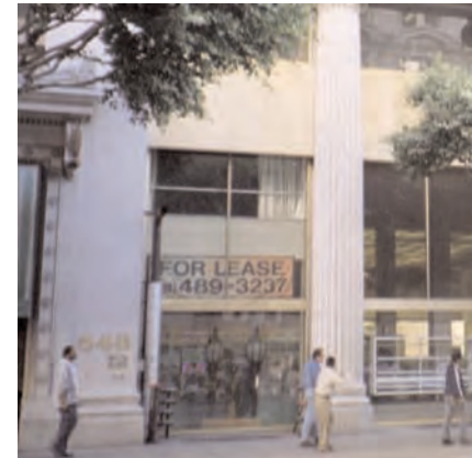
A dropped ceiling above the “for lease” sign is visible through the storefront windows. This diminishes the intended scale of the building and creates visual clutter.
