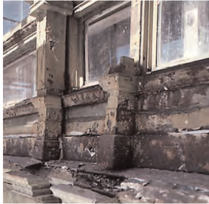
Deteriorated exterior painted surfaces frequently contain lead, which should be professionally abated.
