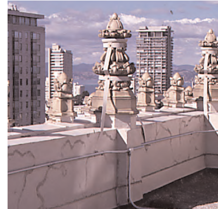
Stabilization of roof top ornamental elements should be undertaken immediately to ensure safety of pedestrians below.
