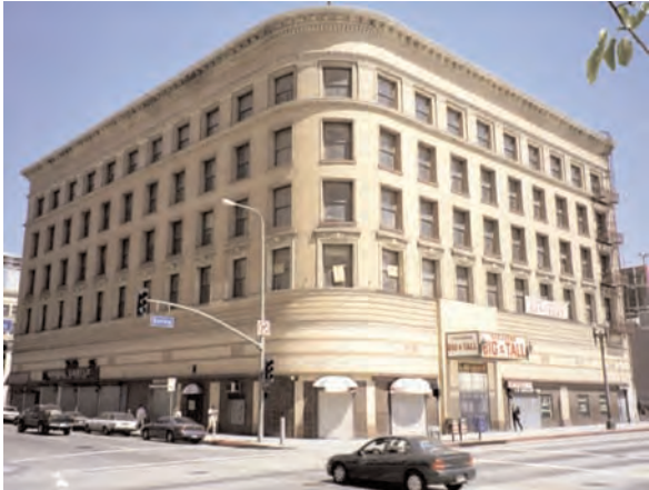
The prominent curved corner of the building is one of the Douglas Building’s most important features. Its reuse should highlight this element of the building’s design.
