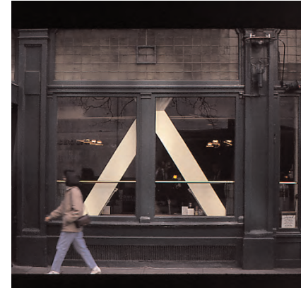
The X-bracing at this storefront has become an important, yet negative, facade element.
