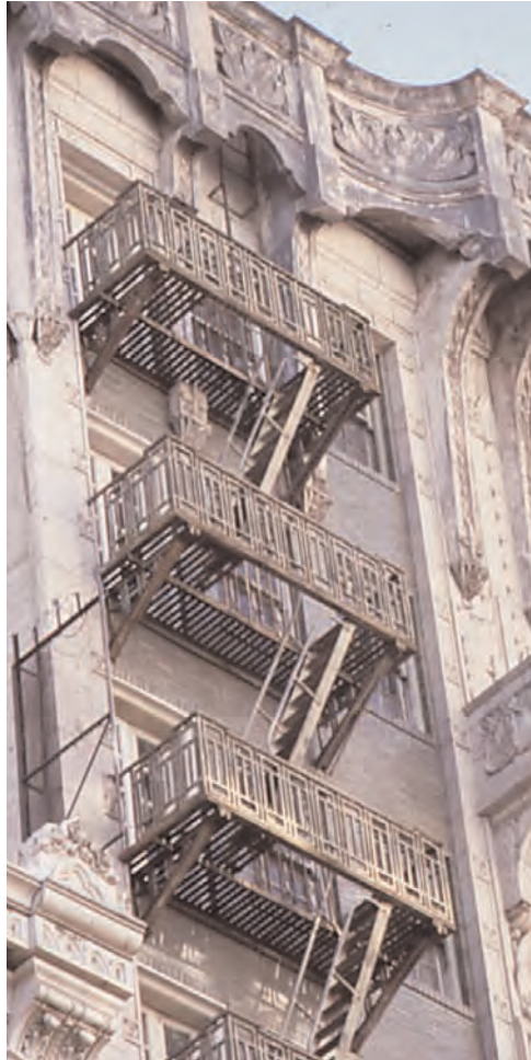
The above fire escape, though not as decorative as the one shown on the previous page, is a character-defining feature of this facade.
