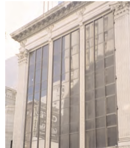
This building has tinted replacement windows that diminish the intended lightweight nature of the structure.
