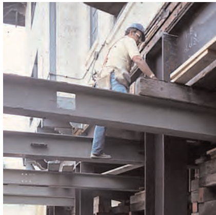
Any unstable condition should be temporarily shored, with minimum damage to the historic building.
