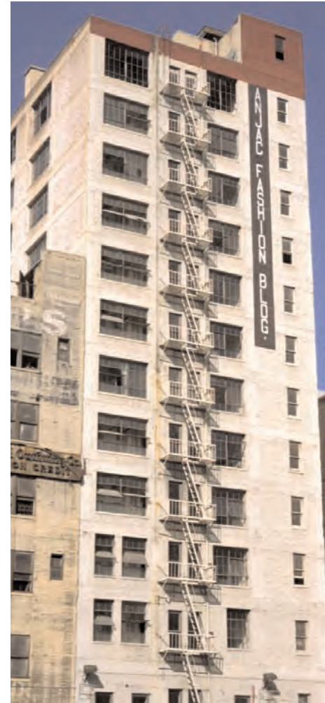
Rear facade materials and features include brick, painted signage, punched openings, fire escapes, and industrial sash windows.
