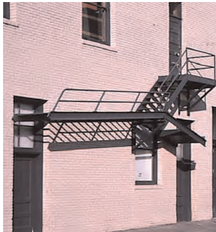
Where they are permitted by code, fire escapes should be maintained in working order.
