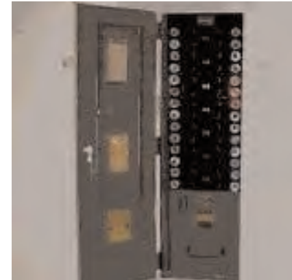
Older electrical service can be a hazard. Note the old fuse system in this photograph. A modern circuit breaker system will likely need to be installed in this building.
