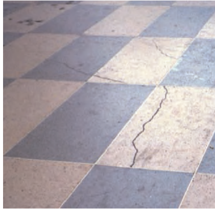
A detail of a cracked terrazzo sidewalk within the study area. While some terrazzo is highly decorative, other elements are composed of simple repetitive patterns.
