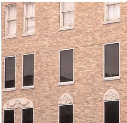
A detail of the original windows above and the replacement windows below.
