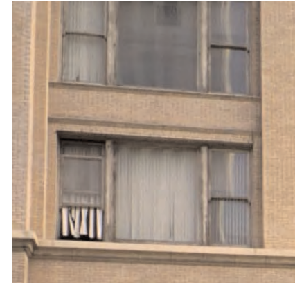
The Chicago Style windows of this building are in need of cleaning and general maintenance repairs.
