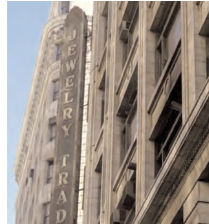
The Jewelry Trades building sign is metal and it is anchored to the building with metal ties into the terra cotta.
