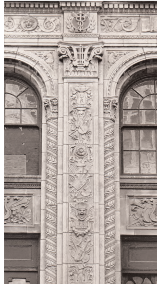
A terra cotta detail of the Wurlitzer Building on Broadway has highly decorative and colorful details.
