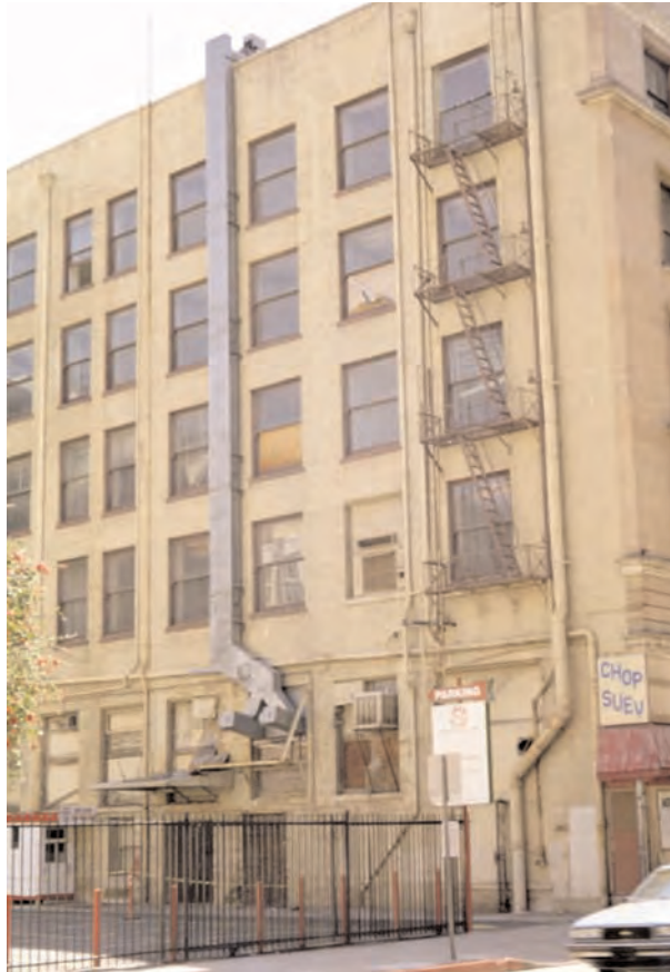
A secondary facade of the Douglas Building, showing the mechanical systems that must be upgraded during a building rehabilitation.
