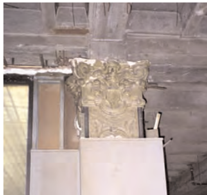
The upper floors of the building were entirely gutted in the 1980s; however, a few original details remain such as this column capital.
