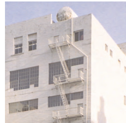
This roof has a large tank visible from the alley behind the building. Tanks of this sort should be checked for hazardous materials. If these elements are obsolete and are not character-defining features they should be removed.
