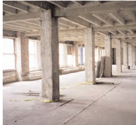
The column grid and the typical windows at the Broadway and Spring Street elevations. The grid could remain exposed in either an office or residential reuse scenario.
