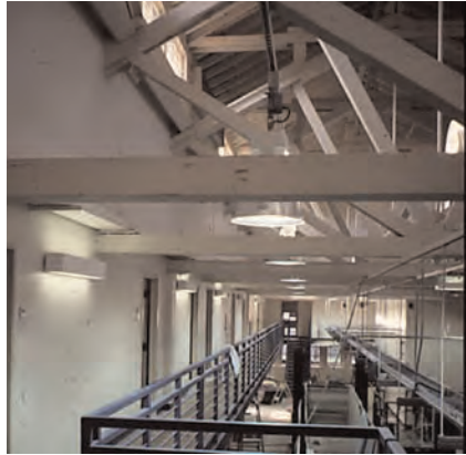
These structural elements are important character-defining features of this building and should be retained.
