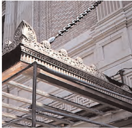
Rehabilitate the area's metal canopies that marked the historic building's original grand entrances.
