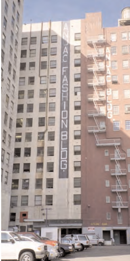
Many secondary facades in the study area are composed of brick, rather than the more decorative material terra cotta.
