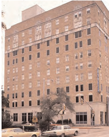
This building has tinted replacement windows that read as dark voids from a distance. This kind of treatment is inappropriate as it greatly alters the facade.
