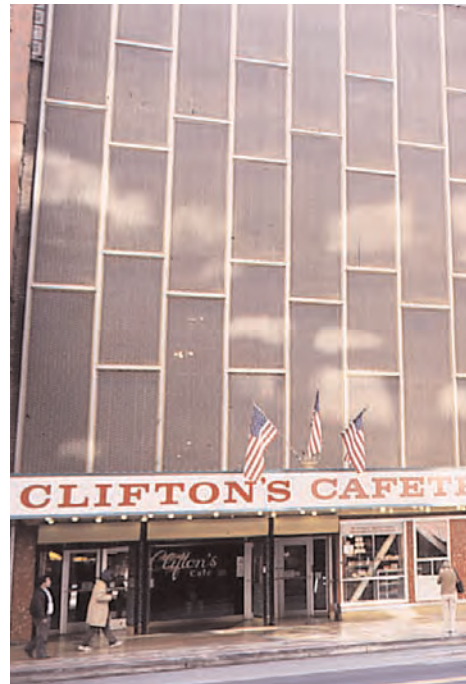
An historic facade is present behind the Clifton's Cafeteria building screen. A rehabilitation project in the future could remove the screen to reveal what is behind, and the features that remain could be rehabilitated and missing features could be re-introduced.
