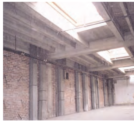
Typical interior spaces at the upper mezzanine that could be used for either residential or office use.
