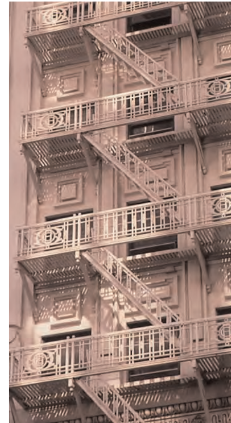
An intricately detailed metal fire escape is one of the most dominant features of this particular building. This element should be retained even if it is no longer used for emergency exiting.
