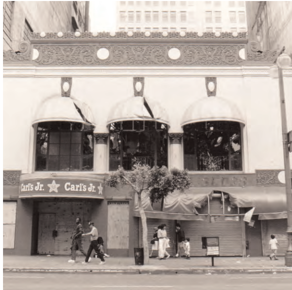
Prior to rehabilitation in the early 1990s, the Victor Dol Building had experienced numerous alterations, including painted terra cotta and deferred maintenance.
