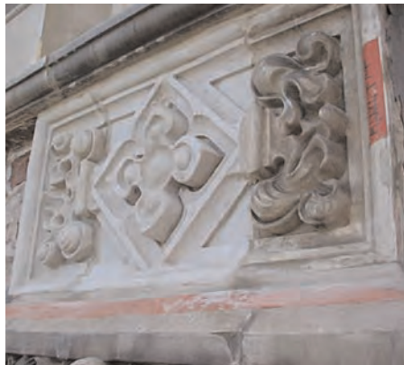
An example of replacement terra cotta elements. Cracking and spalling are common signs of water infiltration with terra cotta. The metal attachments become deteriorated and damage the terra cotta.
