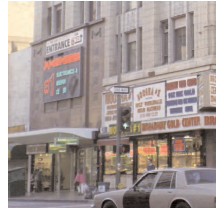
At first glance, the differentiation of materials above the canopy appears to be an original entrance element, but a second look reveals that the sills of the windows above the canopy have been removed, indicating the features are not original.
