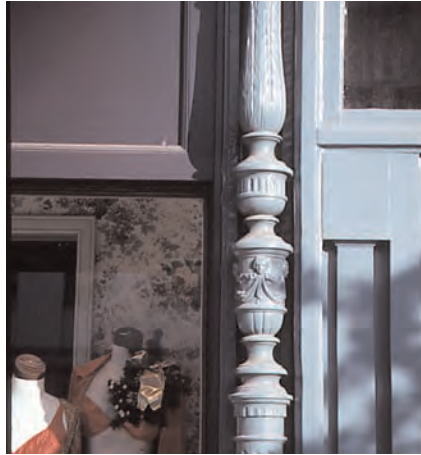
Historic structural elements such as this cast iron column should be retained.
