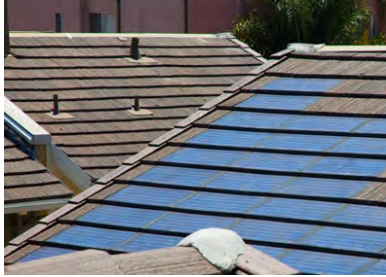
The Gatsby Homes integrate photovoltaic panels into its roof for enhanced energy efficiency.
