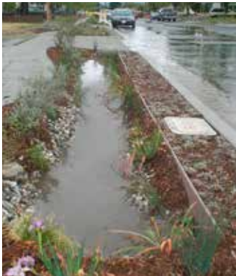
Sidewalk bio-swales treat and reduce runoff {Los Angeles, CA}
